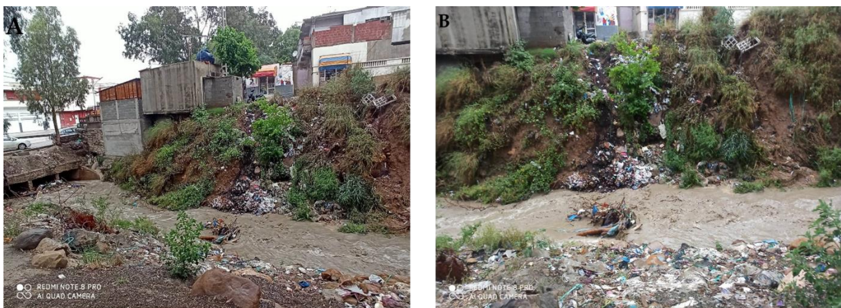
Figure 14. Status of Oued Ziad and causal factors; A) Anarchic urbanization occupying the right bank of the Wadi; B) waste deposited in the minor bed of the Wadi
