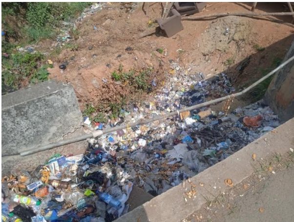
Figure 5: Illegal solid waste dumping along Dick Road, Ibadan
